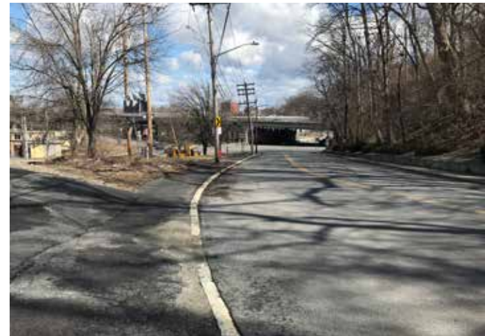
In some areas between Bridge Street and Broadway, private owners have paved over the sidewalk with steep areas of asphalt as a way to reduce the slope in their driveways. This makes the cross-slope steep and difficult to navigate, particularly in precipitous weather.
