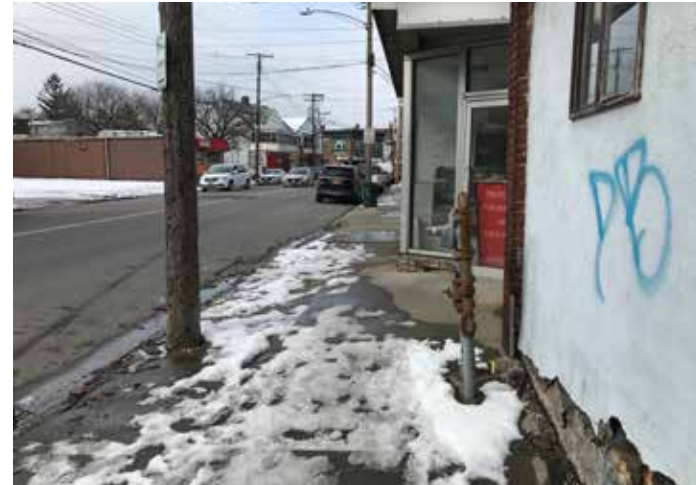
Portions of the sidewalk are very narrow and sometimes cluttered with utilities. This photo was taken between Main Avenue and Francis Avenue.
