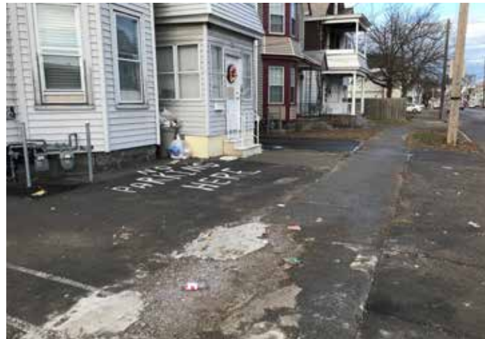
This section of sidewalk between Brandywine Avenue and Steuben Street longer has been partially paved over with asphalt that is now deteriorating. Parking on sidewalks is such a problem that this resident has painted a “no parking message” on the asphalt-covered front yard setback.
