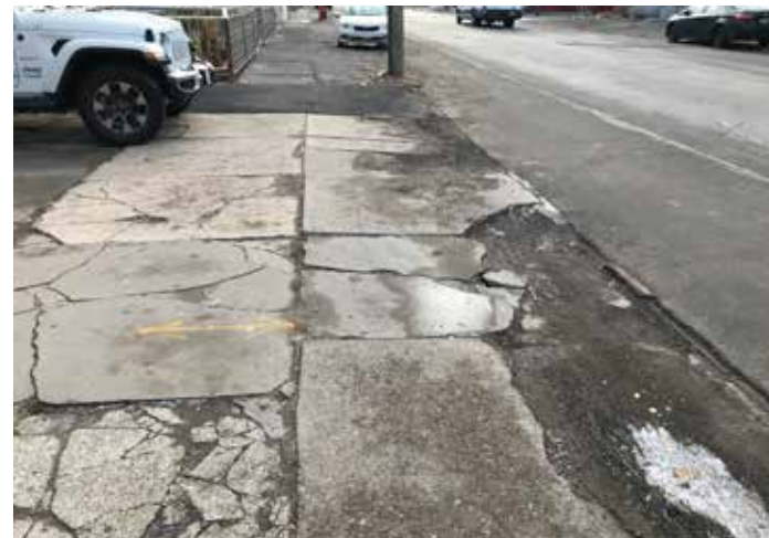
In some area, the road has been paved higher than the sidewalk, and when combined with the poor condition of the sidewalk, this leads to drainage conflicts and pooling of stormwater in walking areas. This photo was taken on Albany Street between Brandywine Avenue and Steuben Street.
