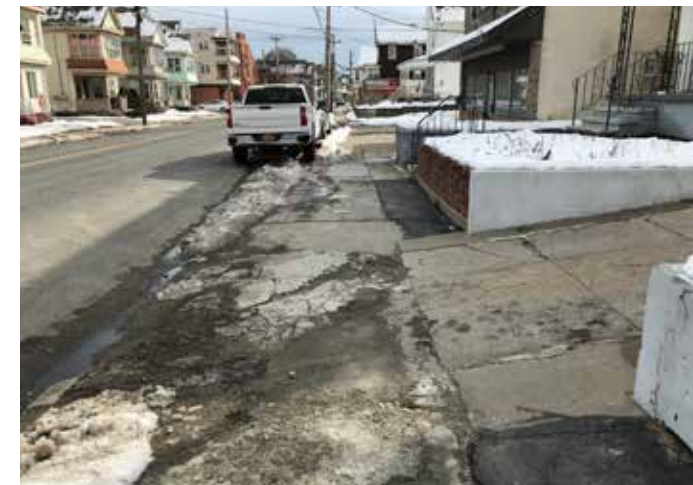
Many areas like this one between Main Avenue and Ostrander Place have severely deteriorated sidewalks.
