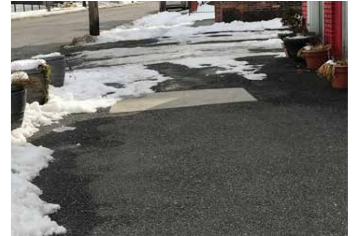
This section of sidewalk has been paved over with asphalt and the business owner is using planters to prohibit parking on the sidewalk and visually enhance the corridor. New sidewalks are often cost prohibitive for small, local businesses and area residents. This photo was taken between Main Avenue and Ostrander Place.
