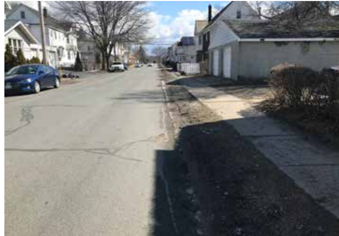
Tire tracks can be seen throughout the tree lawn where the curb is almost gone and cars routinely drive and park.
