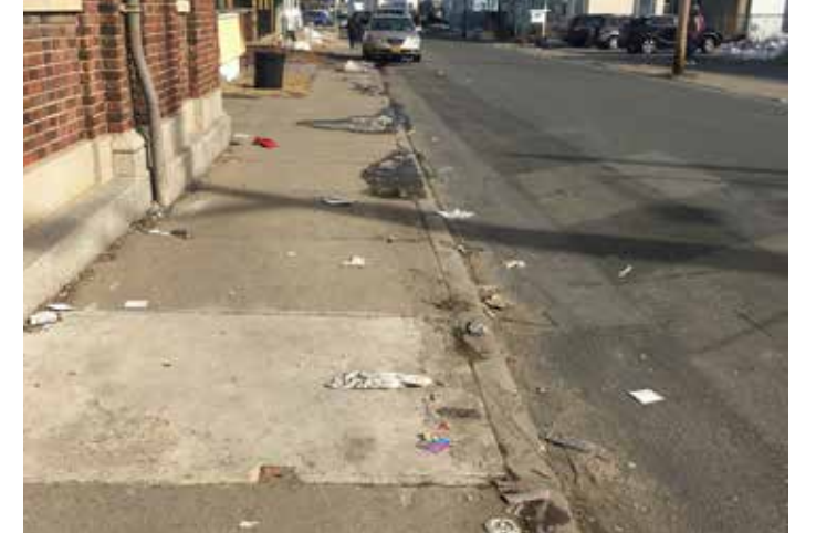
The sidewalk zone on the north side of Main and closest to the Crane / Main / Chrysler intersection is very narrow with no vertical buffers. As seen here, litter is a common occurrence near the commercial core of Crane Street.
