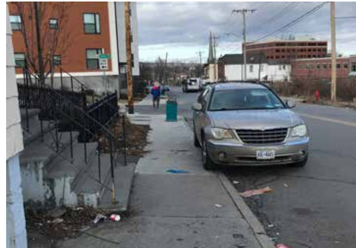
There are some areas where the sidewalk is quite narrow with no buffer to the street edge. Even in situations with higher curb elevations, cars can be seen parked on the sidewalk, making these areas even more difficult for pedestrians to navigate. This photo was taken between Craig Street and Veeder Avenue.
