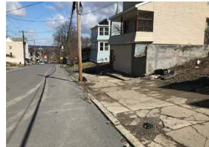
Large portions of the sidewalk are in poor condition, particularly where cars are parking and driving on them. The curb reveal is also largely absent in many locations. This photo was taken in the area between Bridge Street and Broadway.
