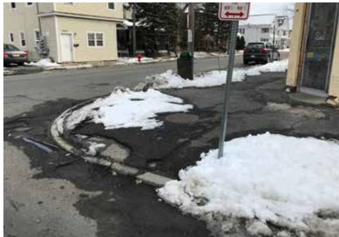
Many intersections are lacking ADA curb ramps and striped crosswalks as shown here at the 6th Avenue intersection.
