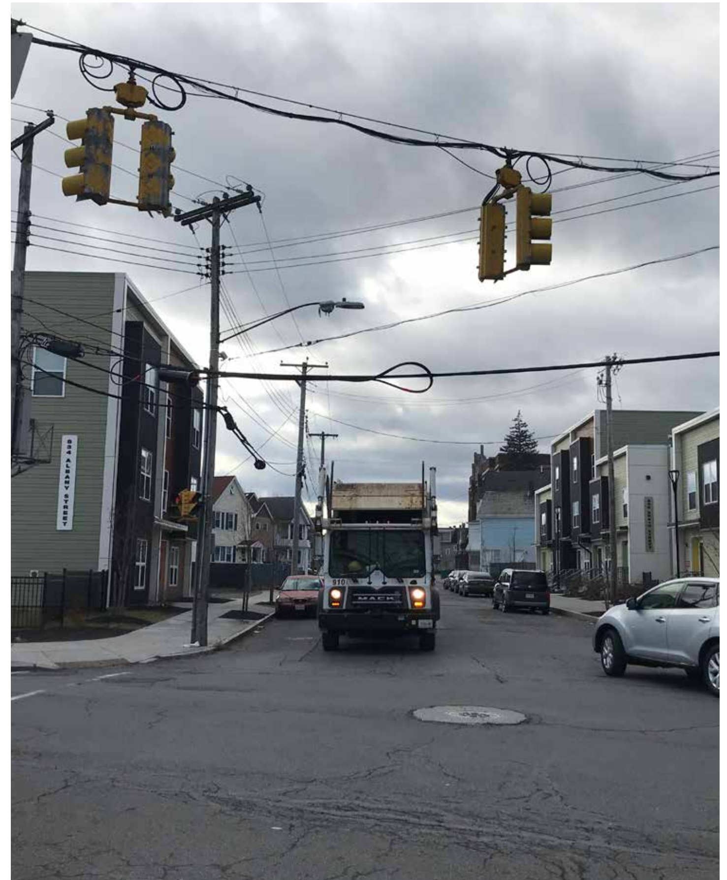
Some ADA access ramps have been added along Albany Street, but much of the crosswalk striping is absent or heavily worn as scene here at the Albany Street and Craig Street intersection.
