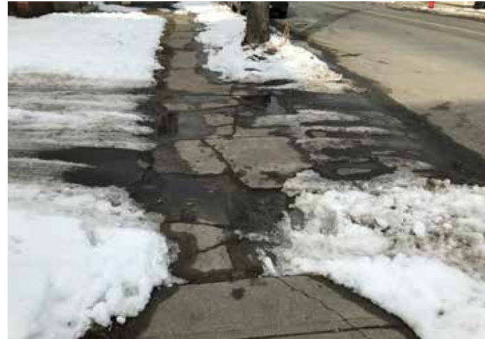
Many of the driveway transitions are in poor condition and make sidewalk use difficult for anyone with walking challenges or pushing a stroller. This photo was taken between Main Avenue and Ostrander Place.
